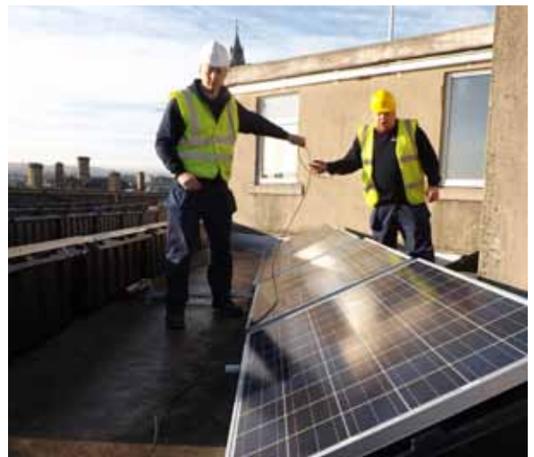
Rooftop solar panels
